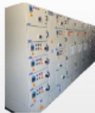
DISTRIBUTION PANELS (630 AMP. MAIN PANEL)
